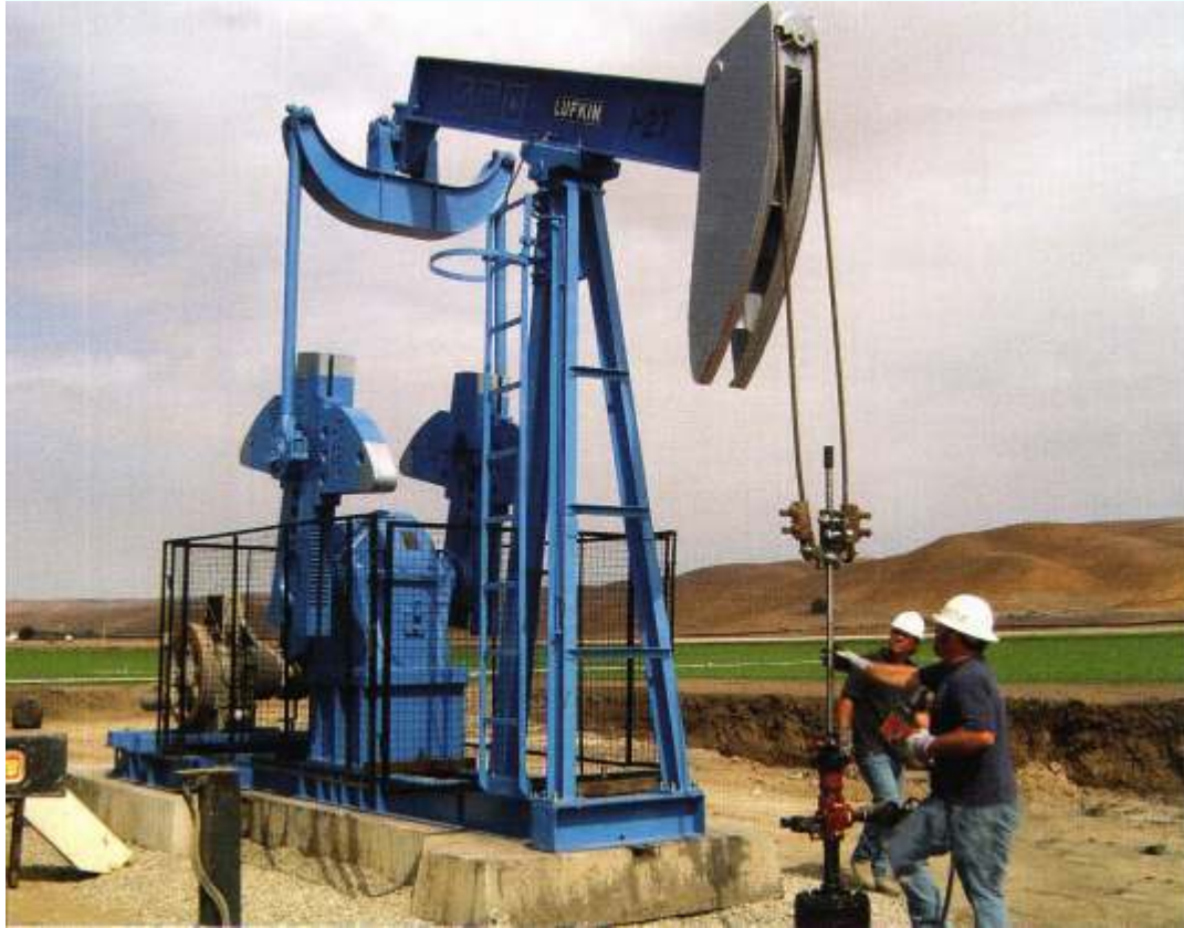
A Salinas Energy well
